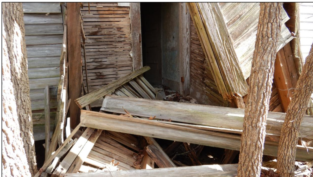
Figure 10. NP0537, dwelling west elevation collapsed entry vestibule, view east.
